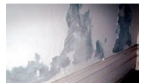
Paint Peel Off
