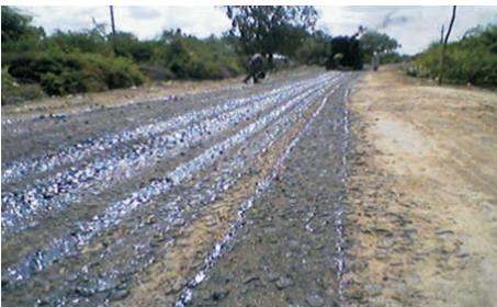
Without Nanotac - Result of Clogged Nozzles
